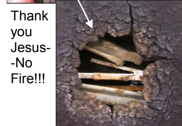
Here is a picture of the breaker box!
